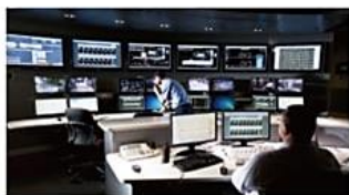
Command and control center
